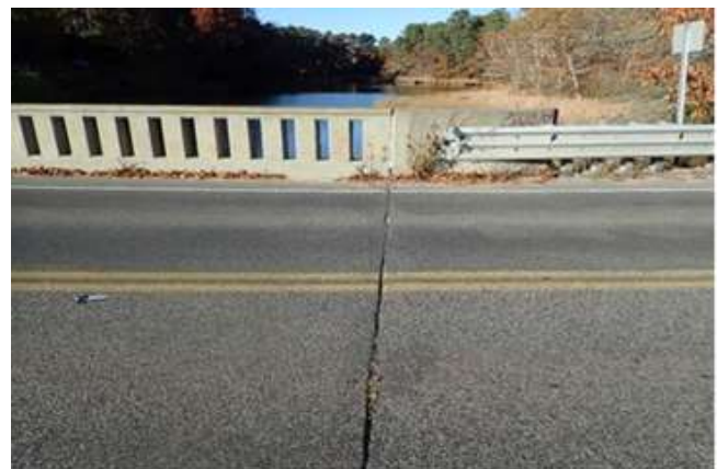
4 Santuit River Bridge joint deterioration
