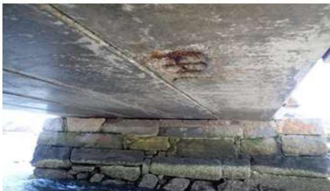
2 Mill Creek Bridge exposed steel reinforcing
