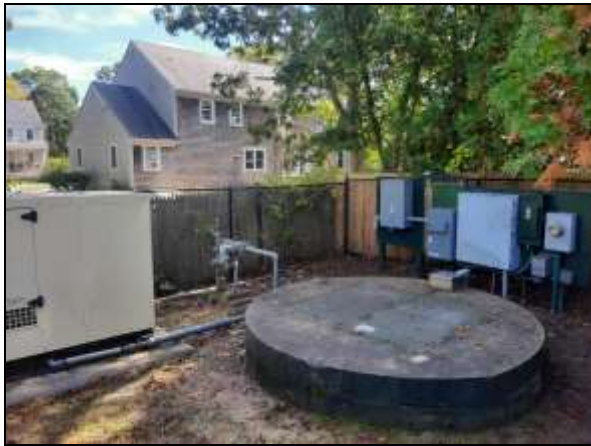
Photo 1: Marks Path Pump Station
