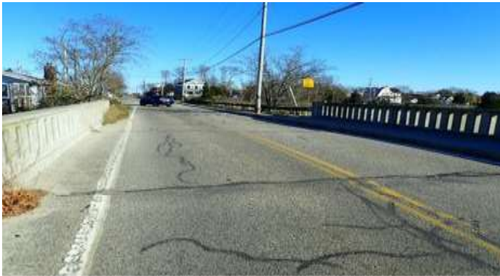
2 Maraspin Creek Bridge uneven settlement
