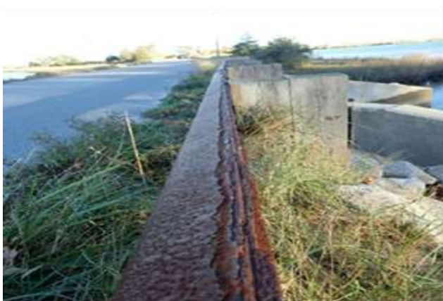
3 Phinney's Bay Bridge guardrail deterioration
