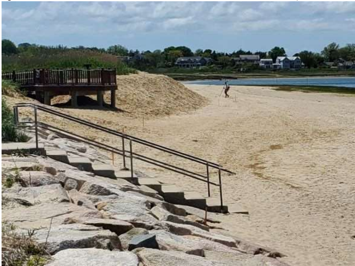
Close up of Post Nourishment with high tide line staked, indicating a narrow work area between the toe of the dune and the high tide line. Also, the high tide line extends up to and within the toe of the adjacent private stone revetment. Picture taken May 2022.
