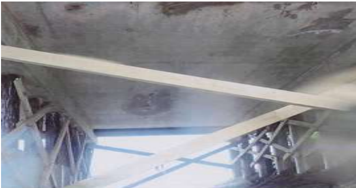
5 Bumps River Bridge some repairs require re-build
