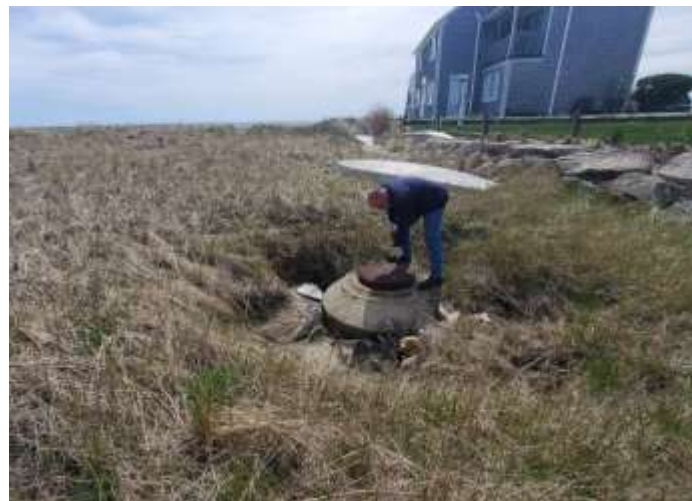
Junction manhole at the connection of an older culvert to a newer culvert that allows saltwater connection to the upgradient salt marsh (taken 3-15-22).
