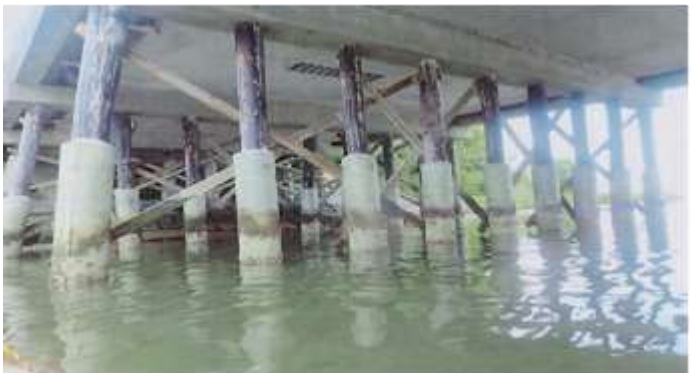
6 Bumps River Bridge some repairs require re-build
