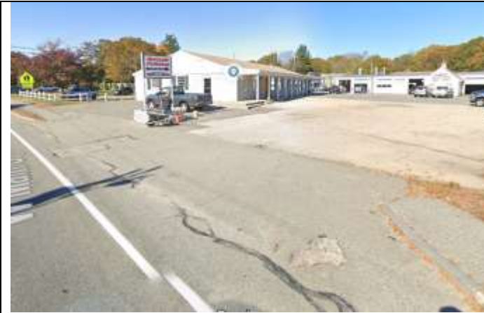
5 Example of excessive driveway opening
