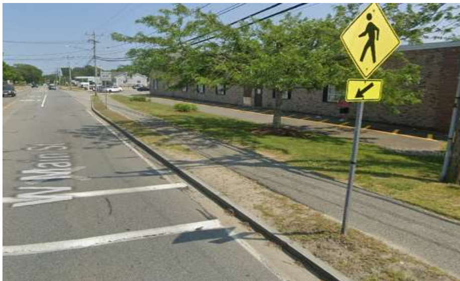
Missing curb ramp
