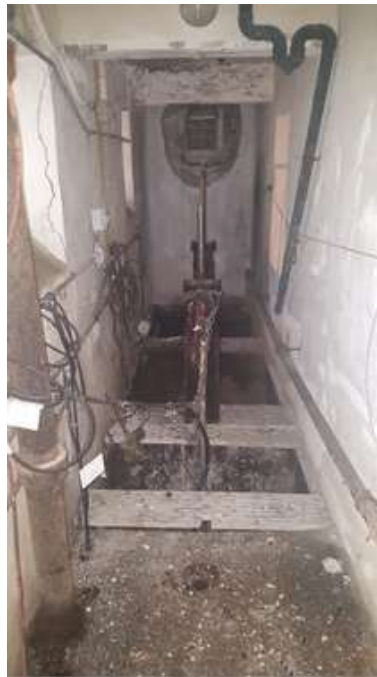
Photo 4: Wet Well Room
