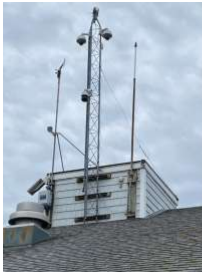
Figure 1 Existing Failed Cameras at Kalmus Beach
