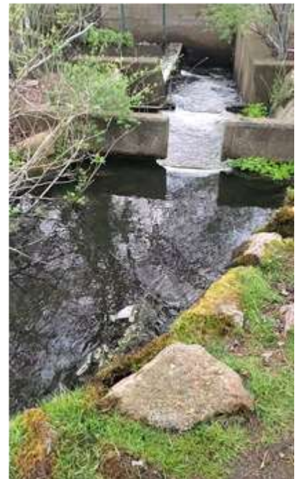
Worn steps and pools along fish ladder.
