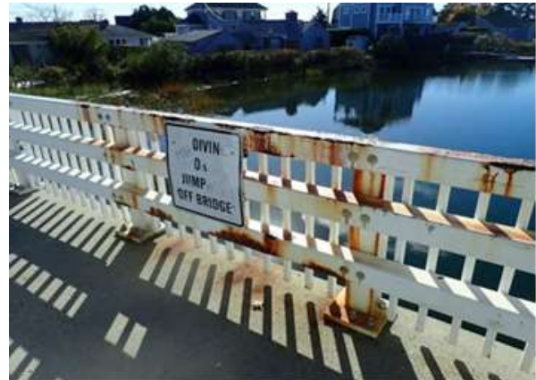
2 Centerville River Bridge rail deteriorated
