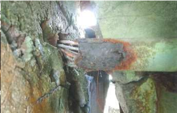
4 North Bay Bridge exposed wires
