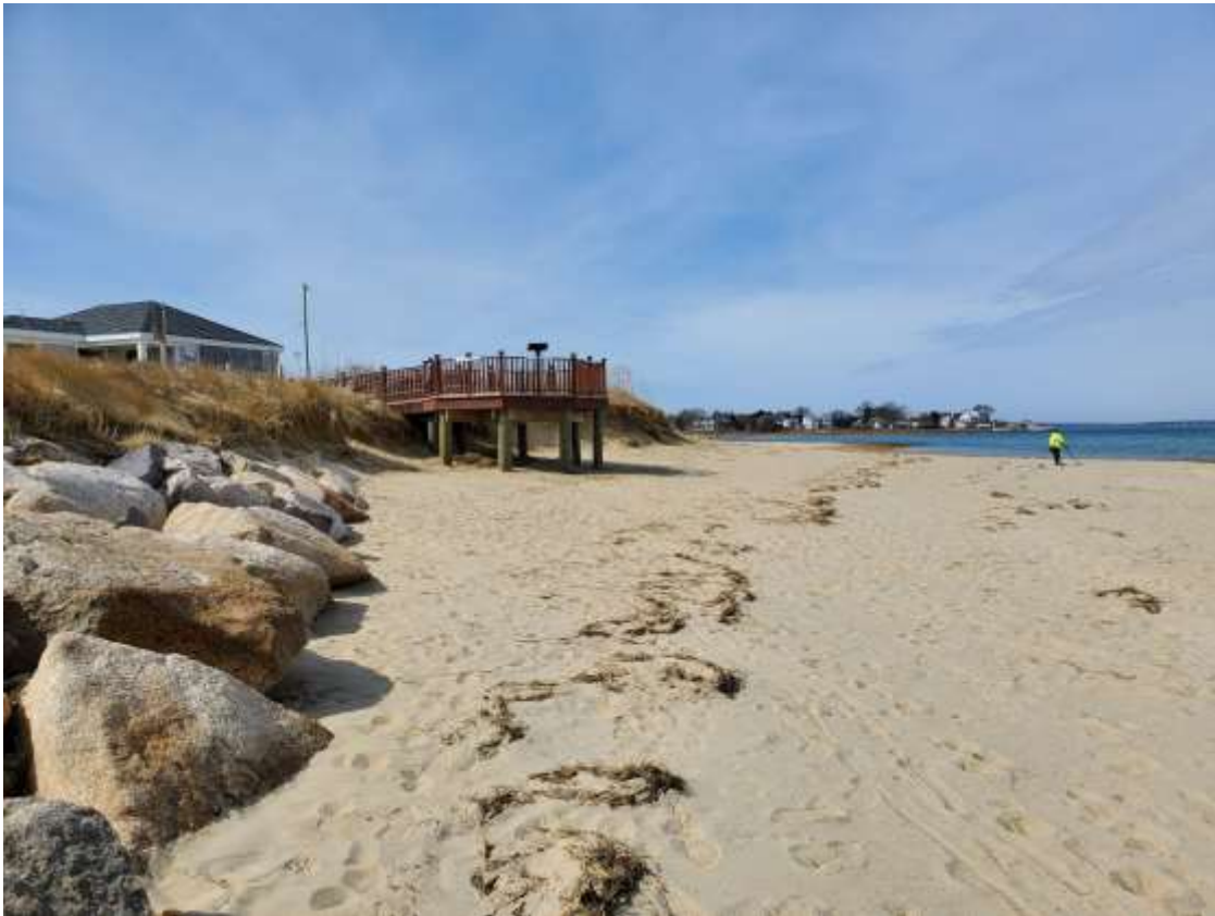
Storm Damage eroded sand underneath the observation deck after Winter Storm Keenan (Picture taken March 2022)
