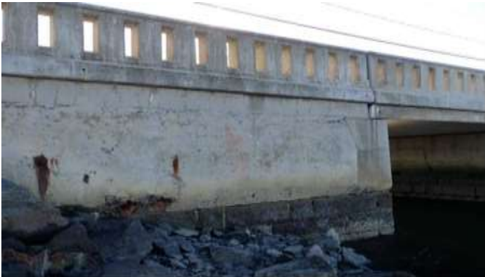
1 Maraspin Creek Bridge deteriorated structure
