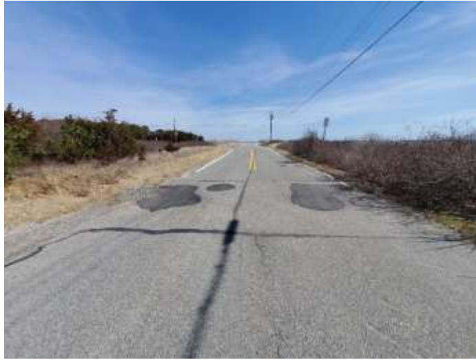
Asphalt and rock patches on Hawes Avenue due to broken culvert pipe under roadway (taken 3-15-2022).
