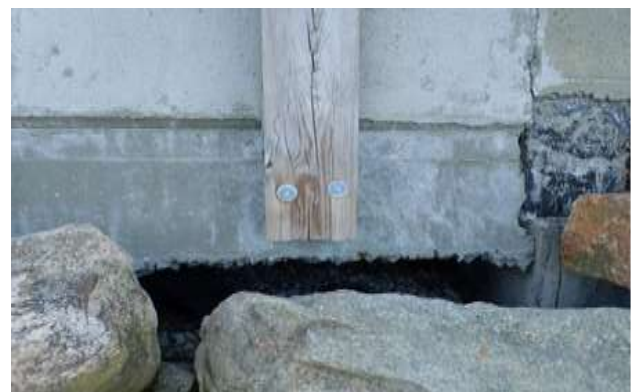
4 Mill Creek Bridge undermining
