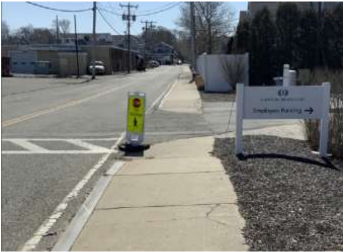
Exceeds allowable cross-slope pitch
