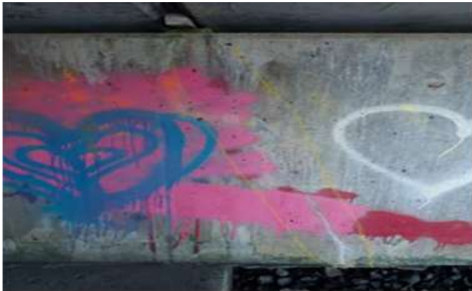
1 Centerville River Bridge beam cracked
