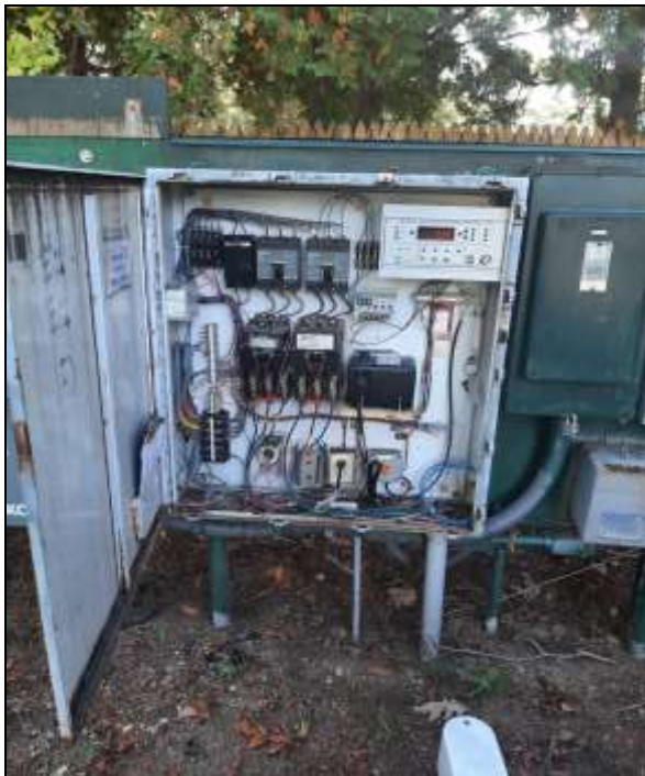
Photo 3: Existing pump control panel
