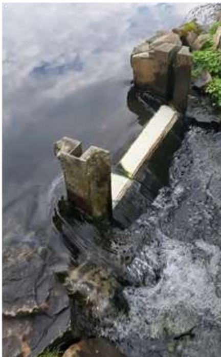
Stone damage and missing stones around the water control structure.
