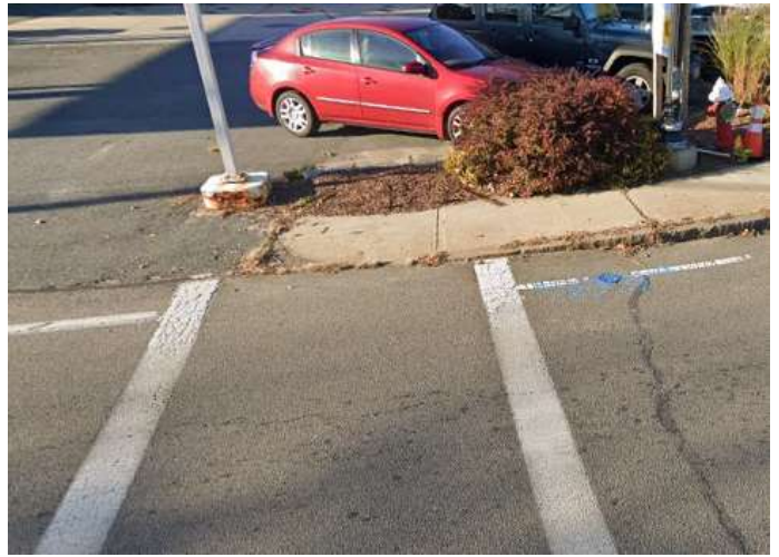
Missing detectable warning
