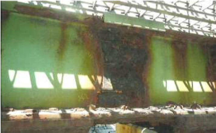
3 North Bay Bridge severe corrosion
